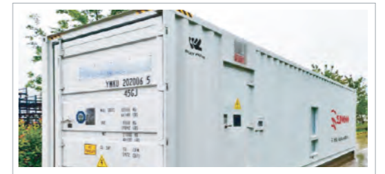
克罗地亚17MWh光储互补项目 Croatia 17MWh Photovoltaic and Storage Complementary Project
