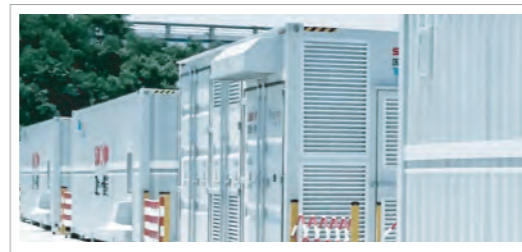
江苏DL工业园80MWh储能电站项目 DL Industrial Park 80MWh Energy Storage Station Project
