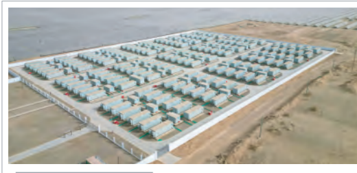
中石油塔里木油田伽师县600MWh光伏发电项目 CNPC's Tarim Oilfield 600MWh Photovoltaic Power Generation Project
